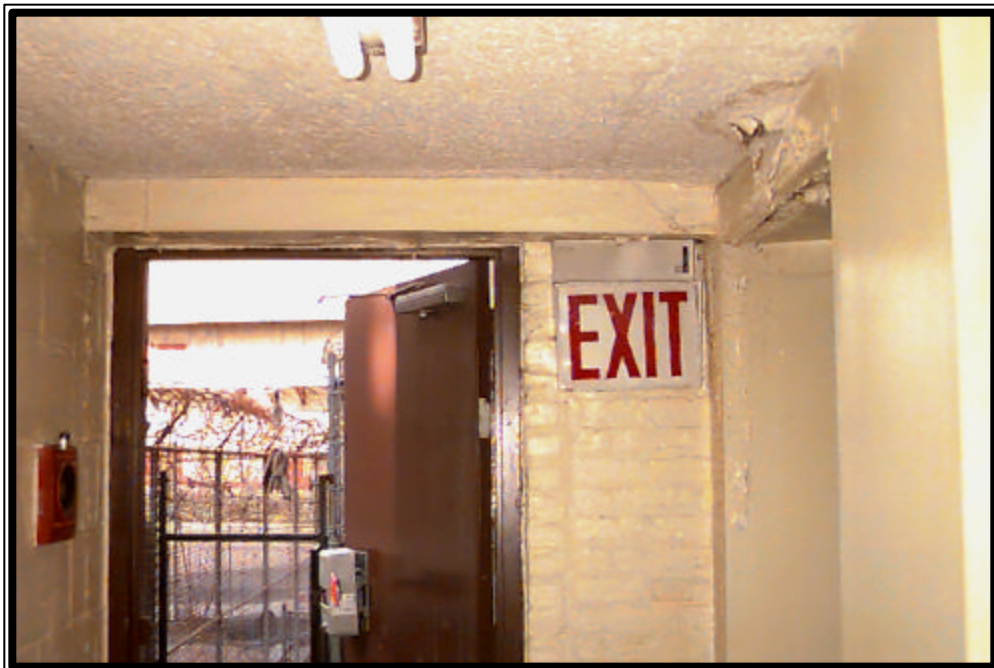
Photograph No. 11 , Damaged ceiling and wall-plaster, and a broken door-closer at Decatur Grant Square Senior Center in Brooklyn.
