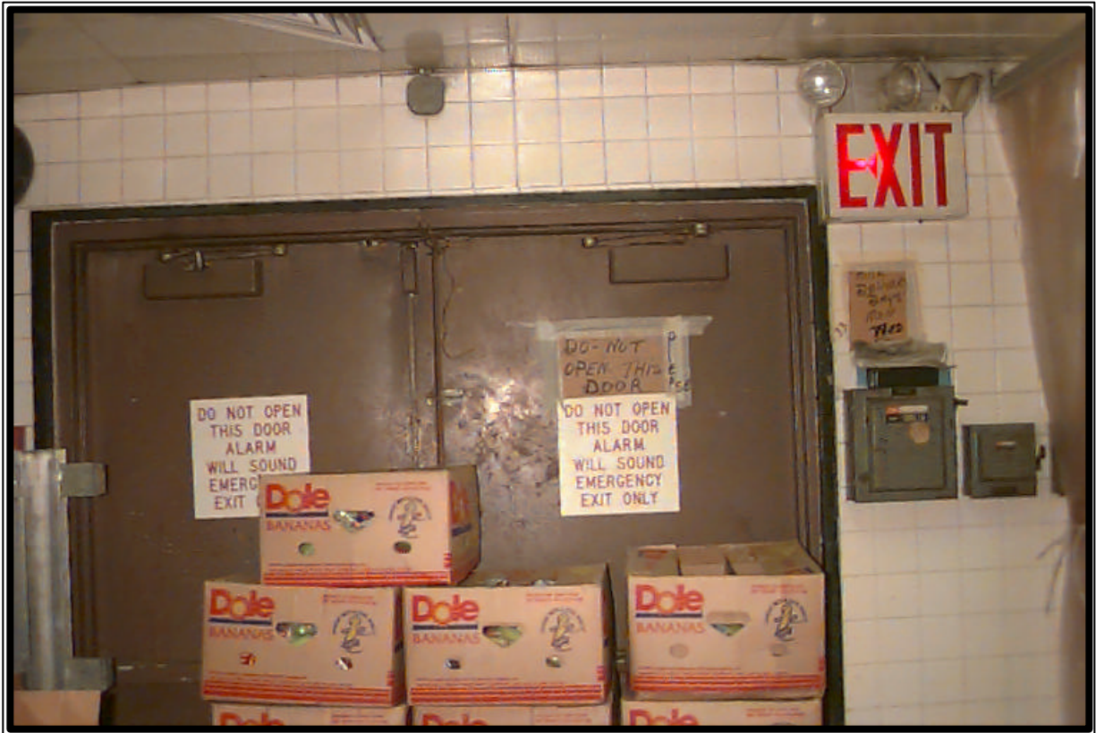
Photograph No. 2, A blocked exit at Brookdale Village Senior Center in Queens.
