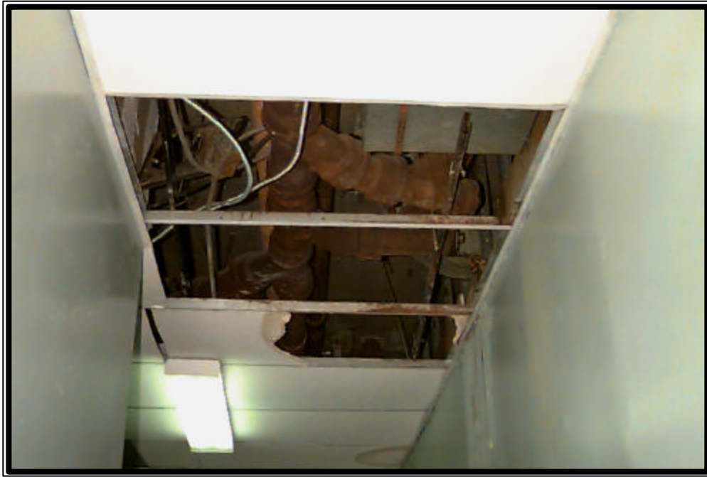
Photograph No. 10 , Missing and damaged ceiling tiles at Schomberg Senior Center in Manhattan.
