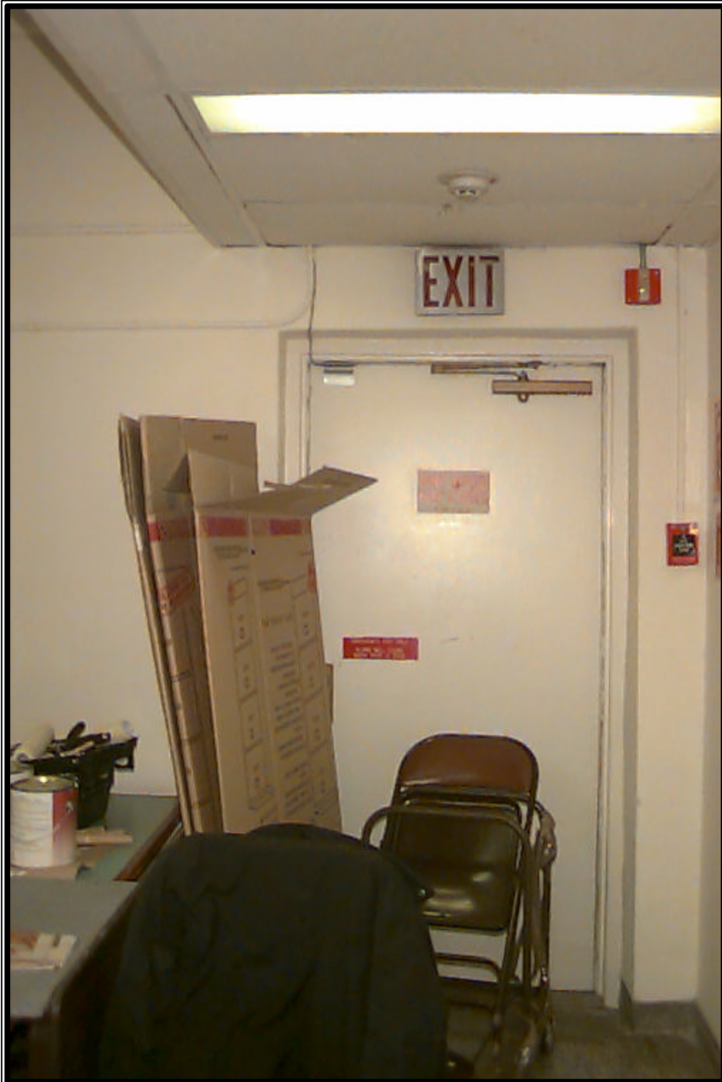
Photograph No. 6, A blocked exit at SNAP Eastern Queens Senior Center.
