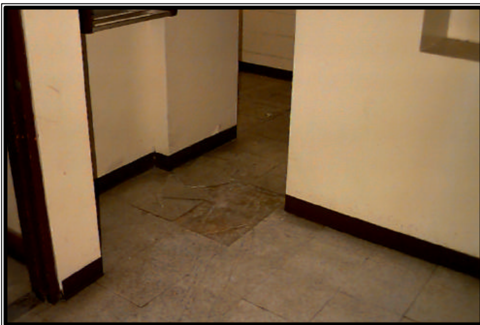
Photograph No. 9 , Loose and damaged floor tiles at Decatur Grant Square Senior Center in Brooklyn.
