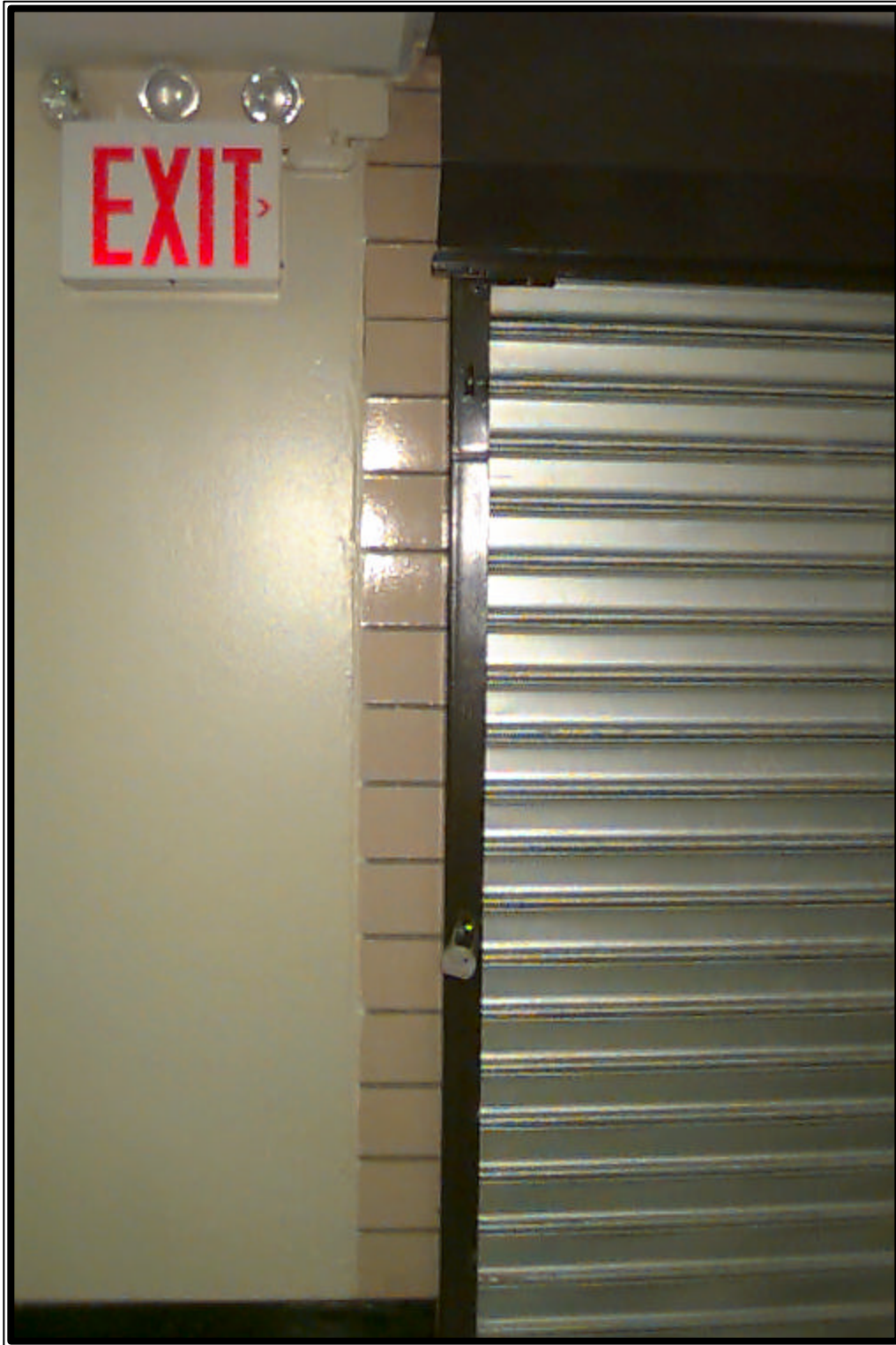
Photograph No. 3, A padlocked exit at Farragut Senior Center in Brooklyn.
