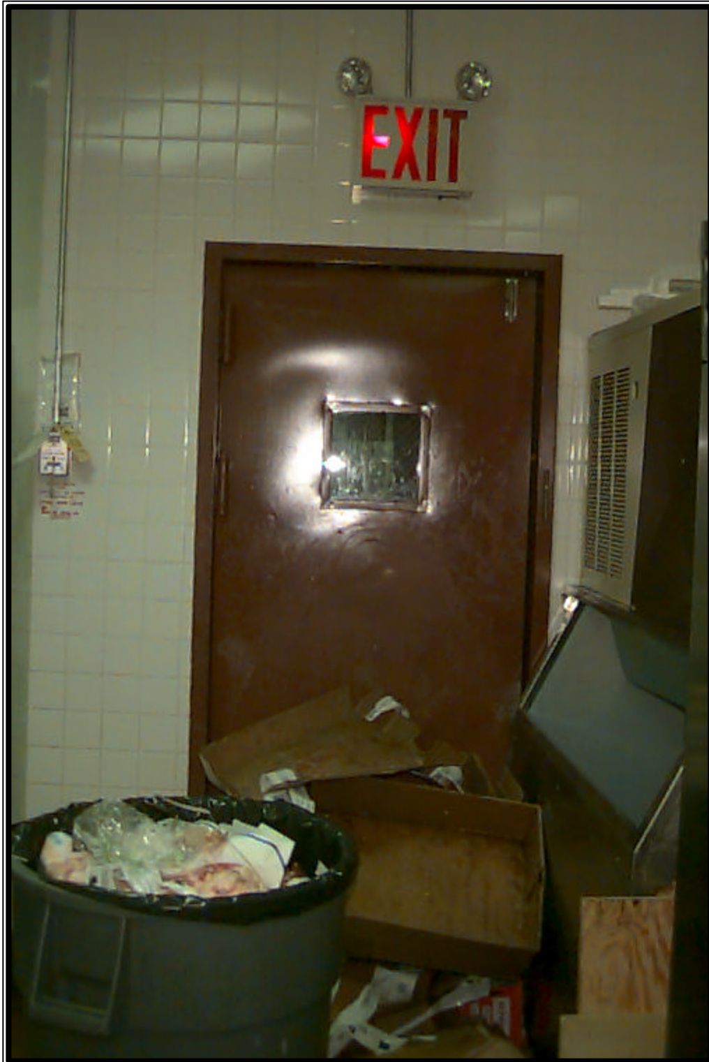
Photograph No. 1, A blocked exit at Sephardic Senior Center in Brooklyn.
