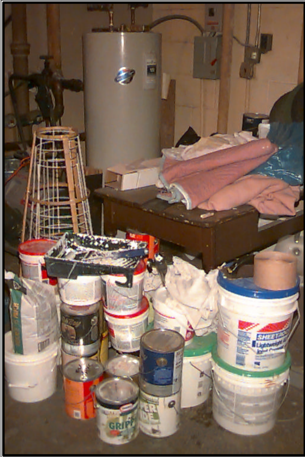
Photograph No. 7, Paint cans and other flammable substances stored near a hot-water heater at Murray Hill SRO Senior Center in Manhattan.
