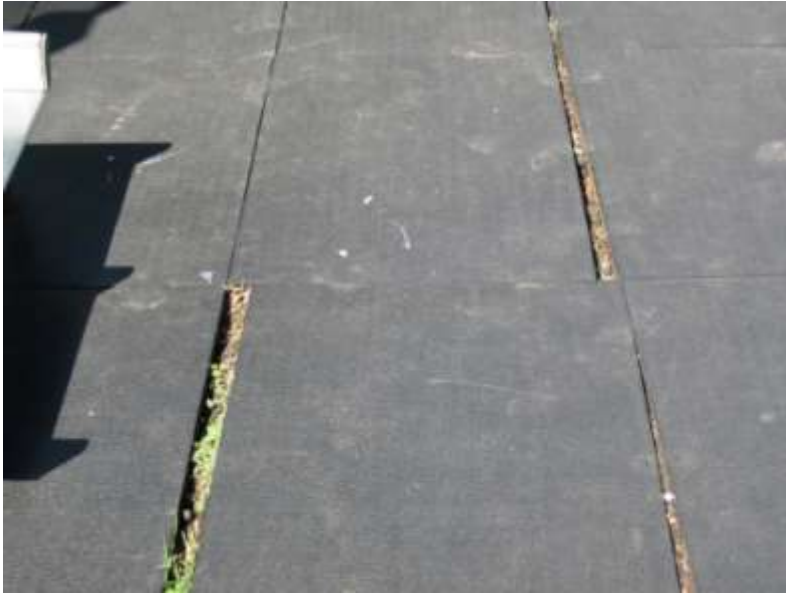
3. Seven Gables Playground Gaps between mats
