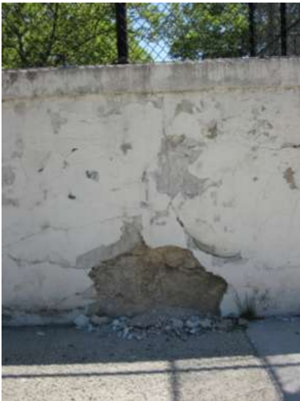
2. Francis Lewis Playgrounds Cracked concrete wall
