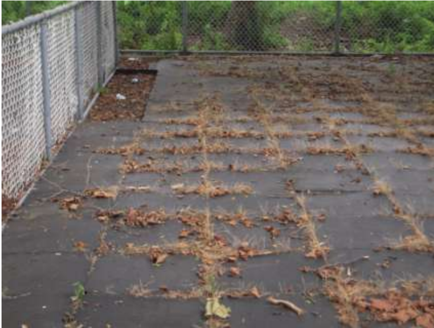
7. Rockaway Community Playground Heavy weeds at play area
