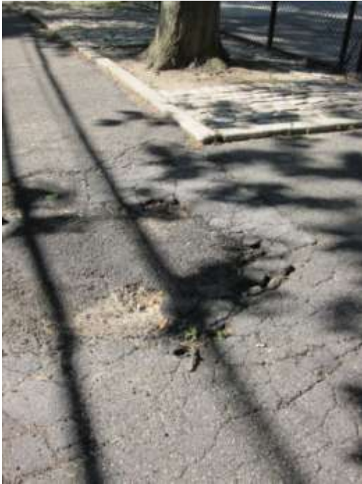
5. Farm Playground Cracked pavement
