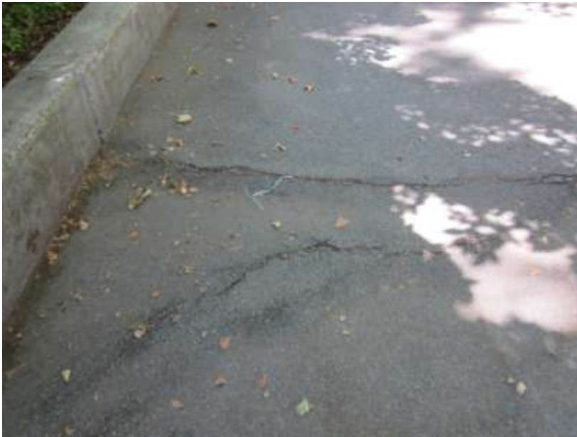
4. Holy Cow Playground Cracked pavements
