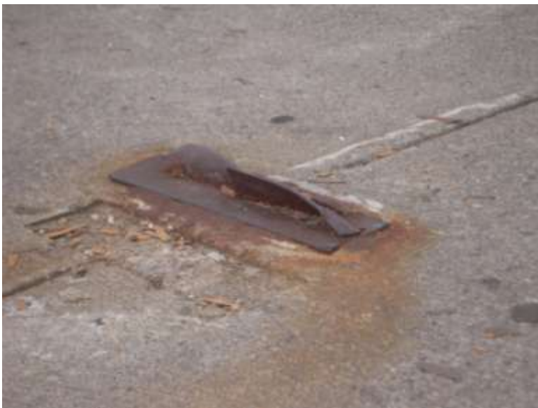
8. Hammel Playground Protruding metal floor bracket at entrance
