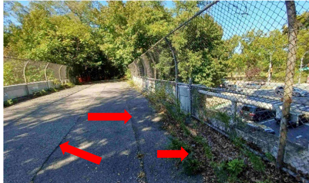
Cracks / Open Joints / Excessive Vegetation
