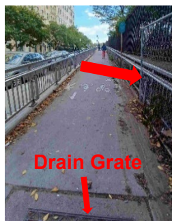
Piece of Fence Blocking Handrail (Right Side)
