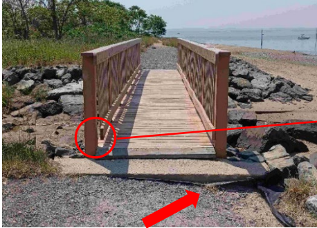
Erosion / Uneven Surface Broken Piece / Disconnected Bottom Rail
