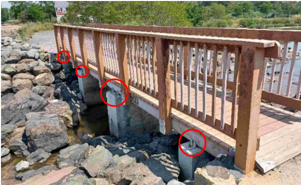
Missing Horizontal Bolt Heads (Entire Ocean Side)
