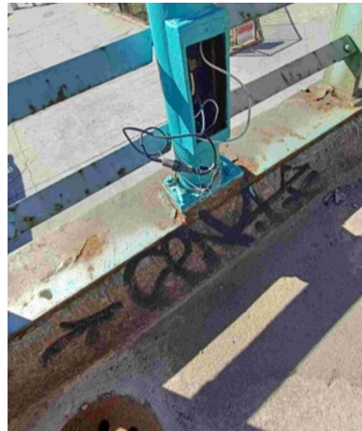
Exposed Electrical Wires
