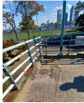
Spalled Concrete / Exposed Electrical Conduit*
