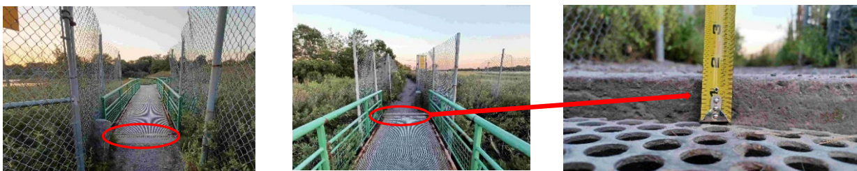
General bridge views (looking north and south). The location of an approximately 1¼-inch drop is highlighted.
