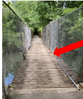
North End Bridge (Not on DPR List) (Inspected and Maintained by DOT) (August 2022)
