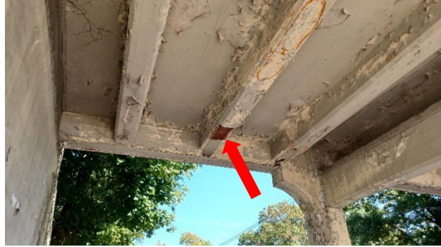
Missing Concrete / Exposed Steel Beam / Peeling Paint Throughout
