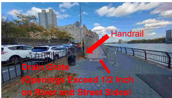
Handrail Does Not Extend the Required Distance Beyond Ramp Run / Drain Grate Openings Issue
