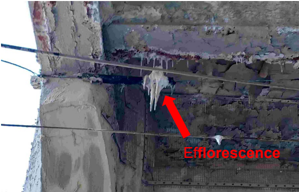
Efflorescence (Indicating Moisture Intrusion Through Bridge Deck Above) / Peeling Paint Throughout
