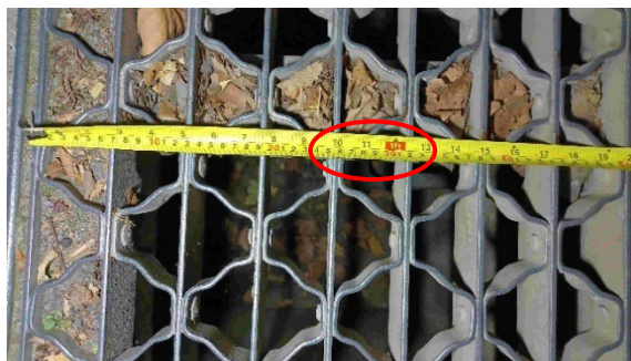
Openings in Drain Grate Cannot Exceed 1/2 Inch per ADA Standards (at Base of Both Ramps)
