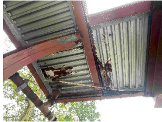
Heavy corrosion (July 2023)
