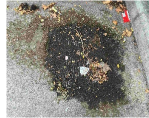
Clogged drain (July 2023)
