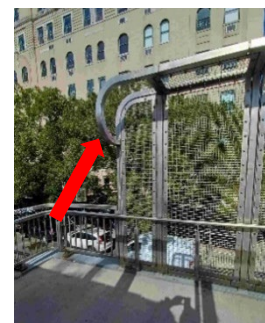
Insufficient Head Room (Below 80 inches)
