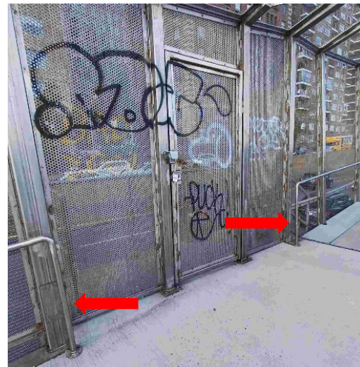
Handrails Do Not Extend the Required Distance Beyond Ramp Runs
