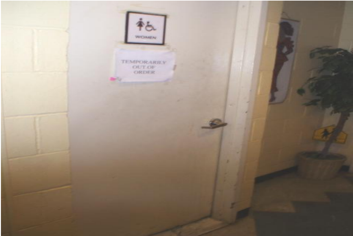
Photograph No. 4– Women’s bathroom out of order at Willoughby Center
