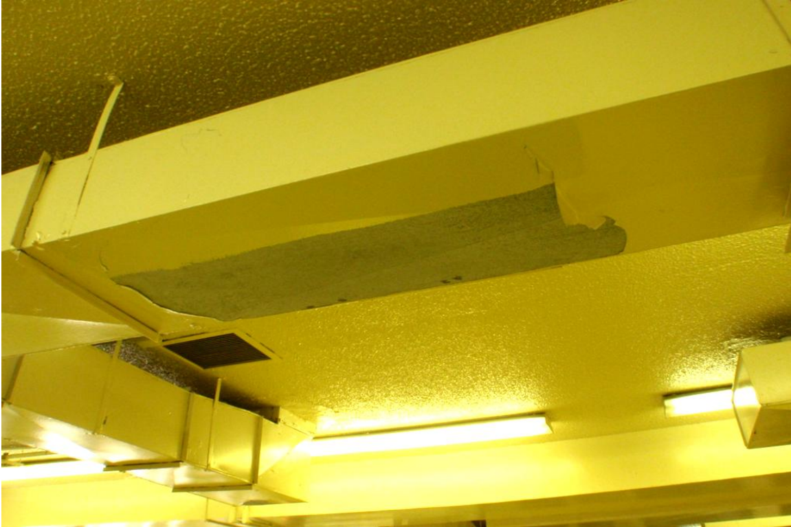
Photograph No. 7 – Peeling paint at CCNS Glenwood Center
