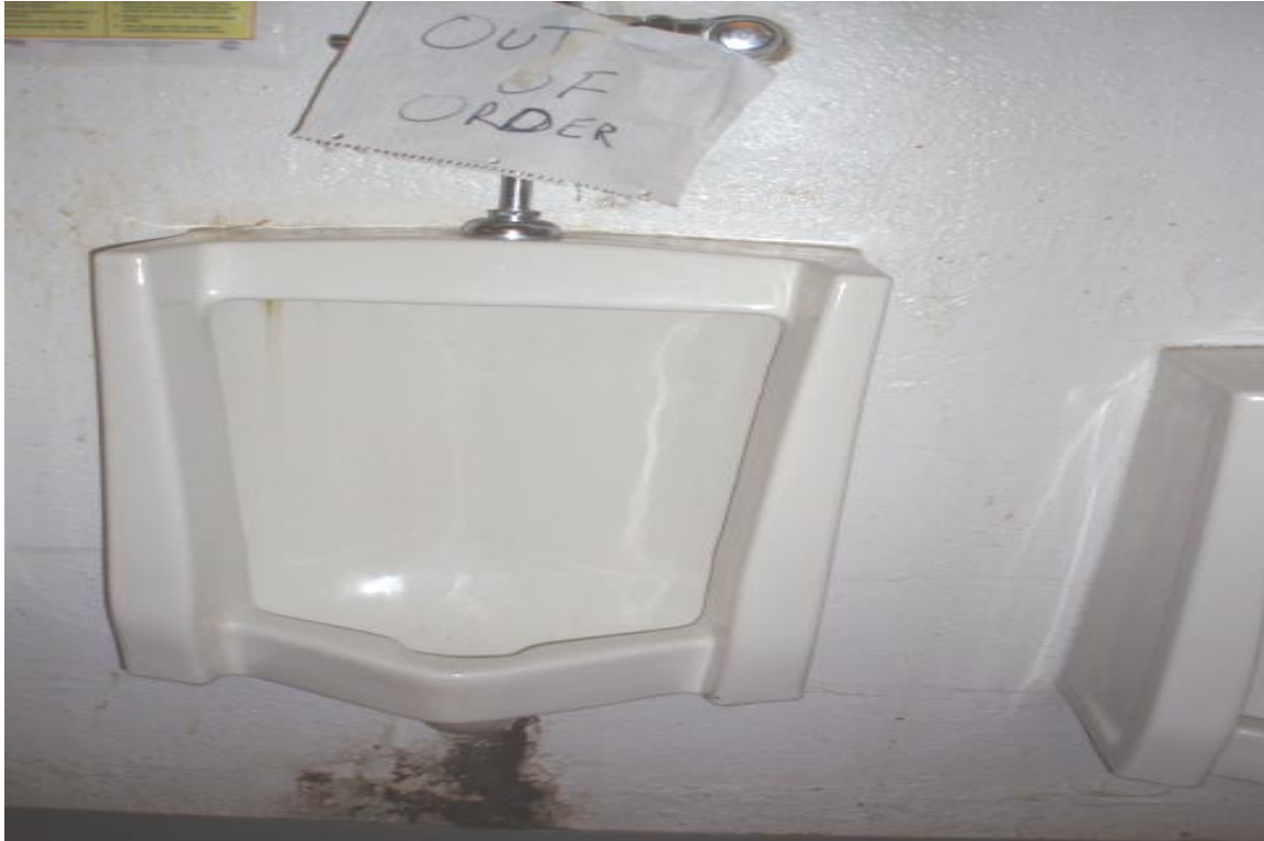
Photograph No. 6 – Out of order urinal at North East Bronx Center
