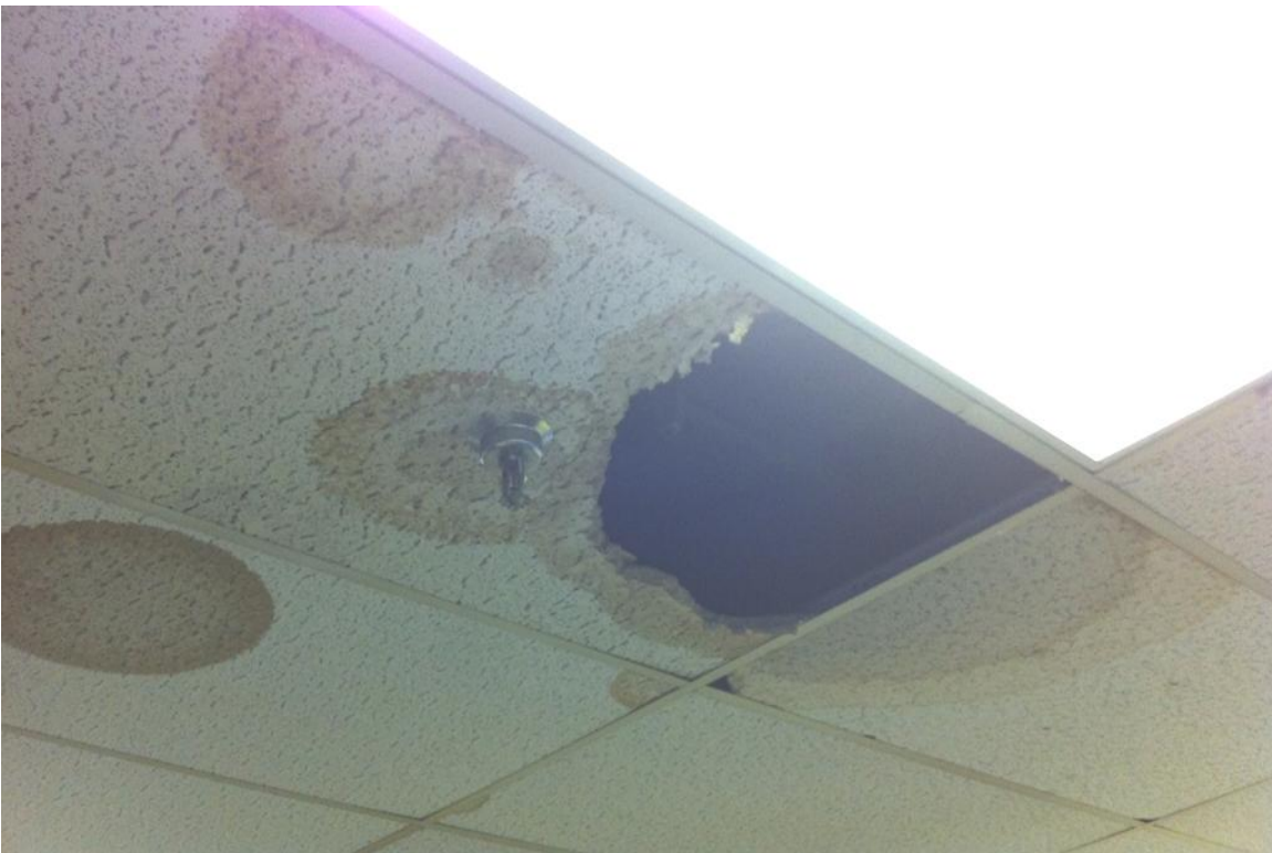
Photograph No. 8 – Water stained ceiling tiles and a portion of one tile is missing at New Lane Center
