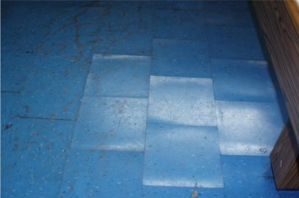
Photograph No. 9 – Warped floor in activity room at West Brighton Center
