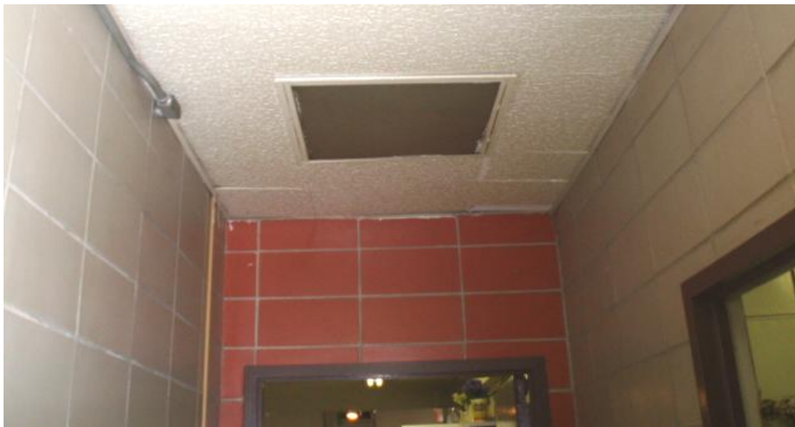
Photograph No.2 – Light out in hallway at Rain Middletown Senior Center
