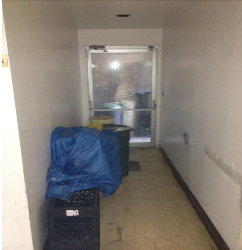
Photograph No.1 – Obstructed exit door at the Korean American Senior Center
