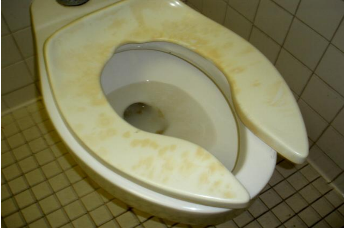
Photograph No. 5 – Dirty toilet seat at Cassidy Coles Center
