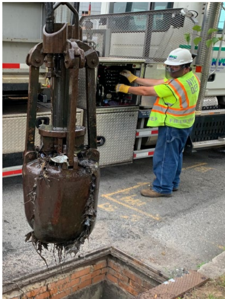
DEP field operations staff operating specialized catch basin cleaning truck. Photo: DEP
