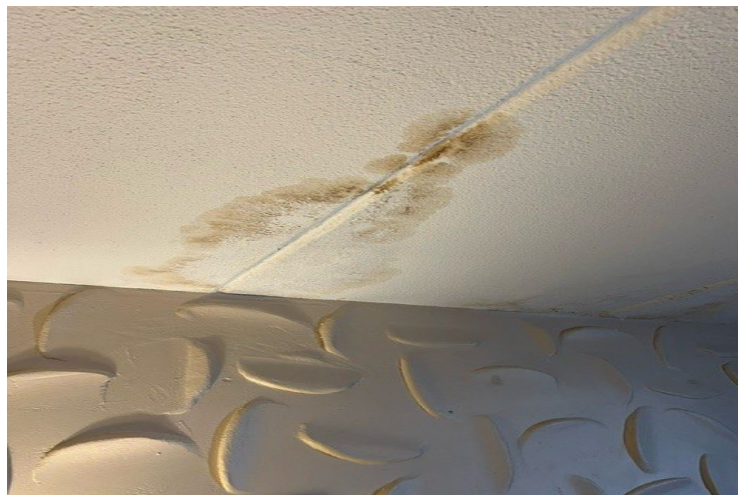
Figure 5: Room 288 had water damage on the bedroom ceiling in two places.
