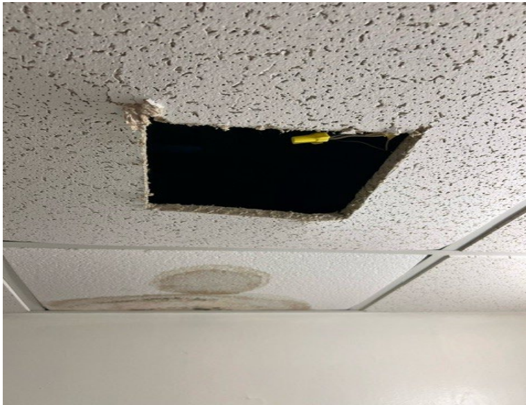
Figure 4: Room 288 had a hole in the bathroom ceiling.
