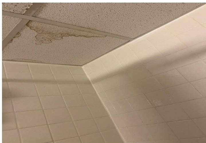
Figure 1: Room 130 had water damage on the ceiling in the bathroom.
