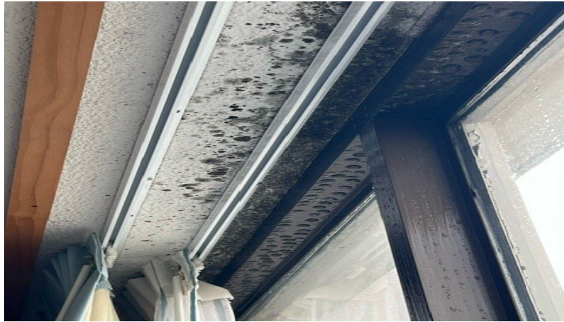
Figure 2: Room 261 had a serious mold problem and the room had a bad smell. Water from condensation on the window was on the windowsill inside the room and the carpet was very wet near the window. Numerous mold spots were observed above the window.
