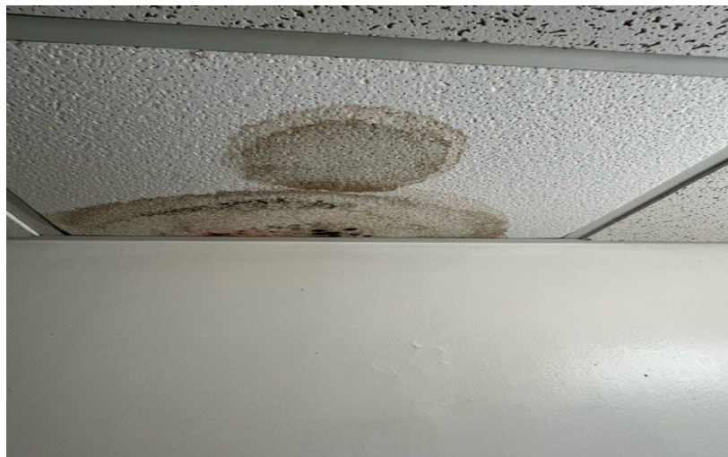
Figure 3: Room 288 had mold, water damage, and a hole in the bathroom ceiling. This room also had water damage to the bedroom ceiling in two places.
