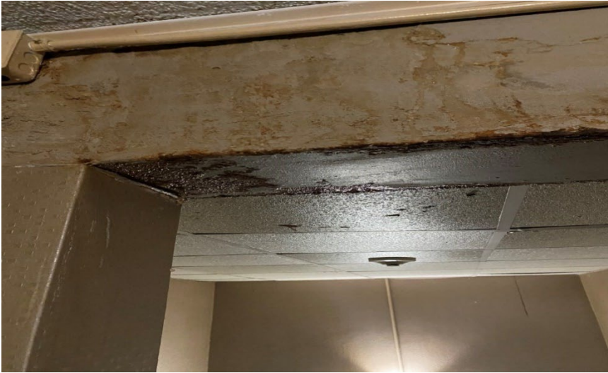
Figures 11 and 12: Ramada Inn, leak in second-floor hallway
