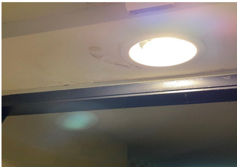
Figure 13: Crossroads Hotel, leak in hallway
