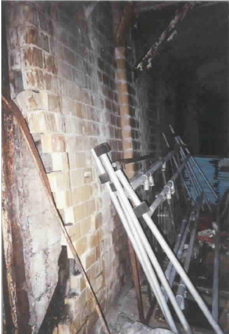
Cracked wall with missing and loose bricks in a condemned section of the Support Service Division storehouse.
