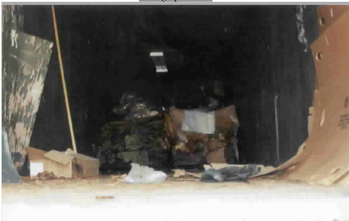
Trailer in need of repair because of holes in the ceiling of the trailer, as shown by light coming through.
