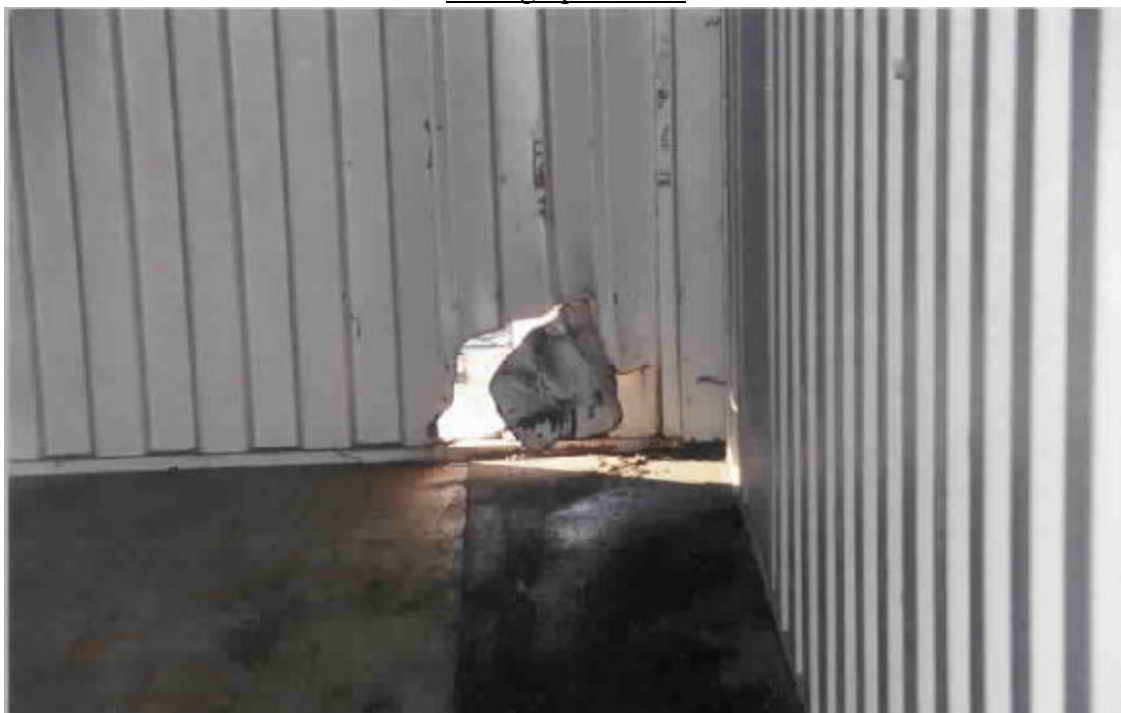
Trailer in need of repair because of torn wall, as shown by light coming through.
