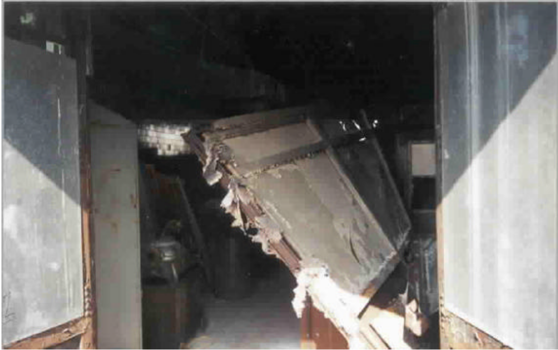
Cracked and torn partition in a condemned section of the Support Service Division storehouse.
